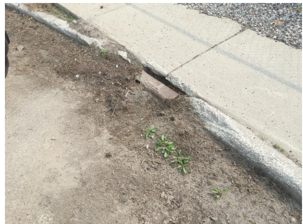
Figure 23 A severe example of a drain on Olson in need of maintenance or LID. Sediment is plugging the storm drain reducing effectiveness.
