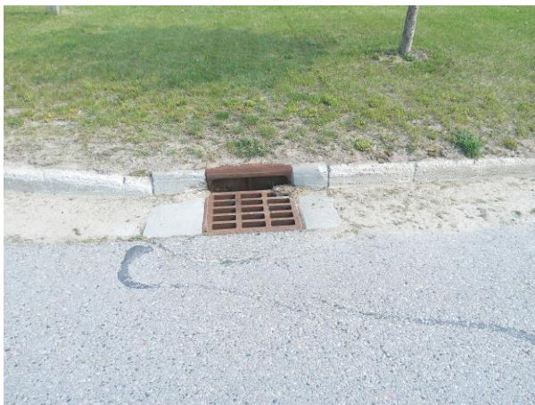
Figure 21 This drain is an example of where street sweeping would capture sediment containing pollutants from entering the storm sewer system. Sand on both sides of the drain will be washed into the storm sewer system during rainfall events, mobilizing both suspended solids and nutrients.
