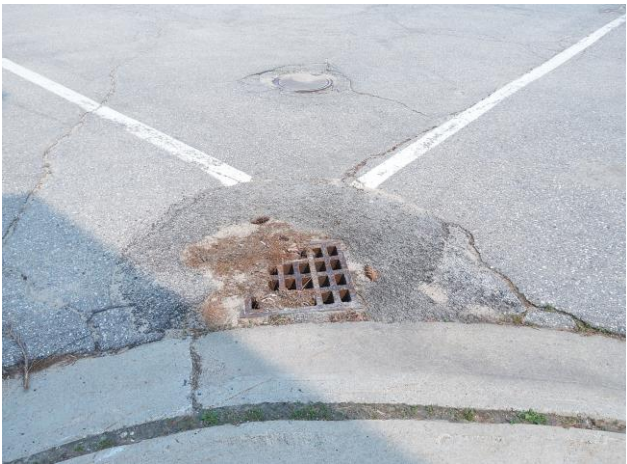
Figure 25. Olsen Street drain and crack with debris.
