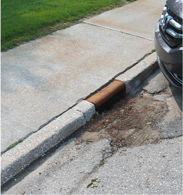
Figure 24 An example of a drain on Kneeland in need of sweeping/maintenance
