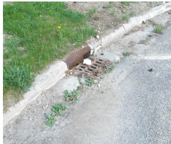
Figure 22 Example of a storm drain on Olsen in need of clearing/maintenance
