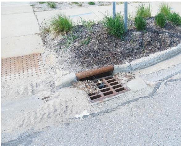
Figure 20 Example of a storm drain at the intersection of Salling and Kneeland that would benefit from strategic street sweeping.
